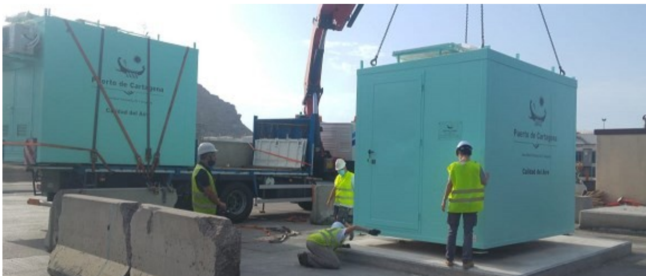
New metering booths
