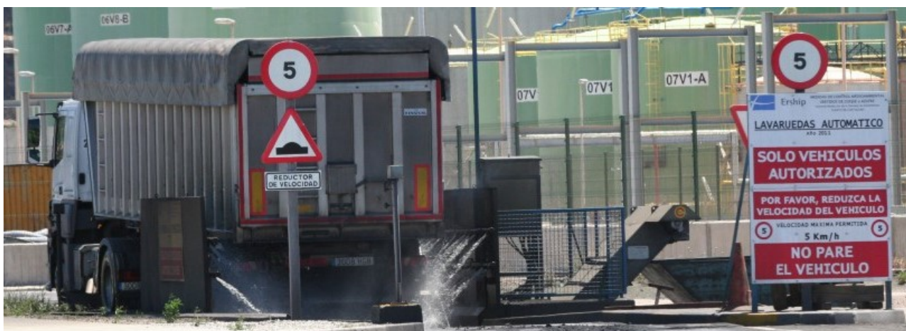
Automatic wheel washers installed at the bulk terminal to minimize dust emissions from transport
